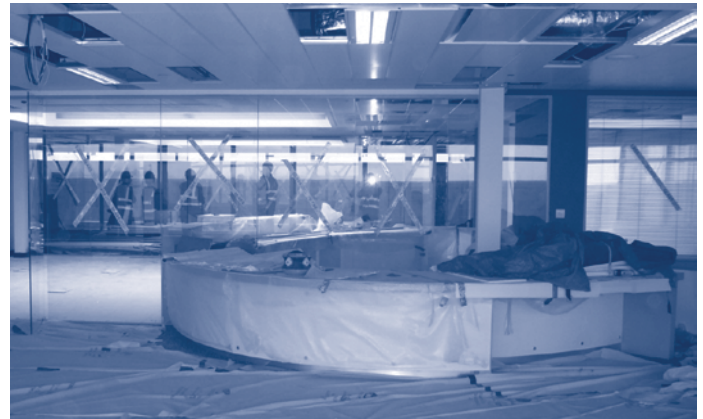
The wraps almost ready to come off from the Level 6 Reception to the new Centre for Research Collections
