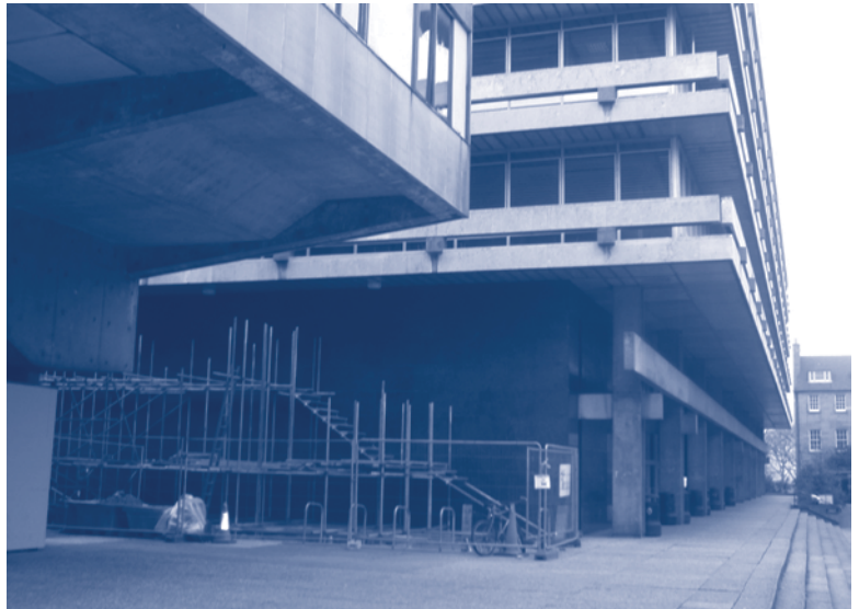
Scaffolding being erected to create steps up to a temporary main entrance to the Library which will be knocked through into the First Floor. An external lift is to be added for users with mobility difficulties; until it is ready, access is via the west door (see below)
