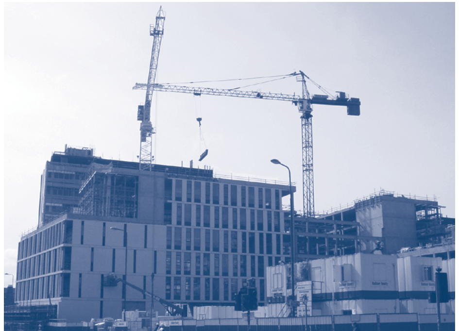
The Informatics Forum taking shape, well on its way to becoming a landmark centre for innovation and interaction. See http://www.inf.ed.ac.uk/building/
