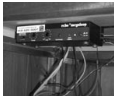
A counter Loop amplifier fitted under the desk
